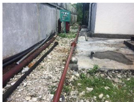
Figure 6. Condition of the existing fuel piping system
